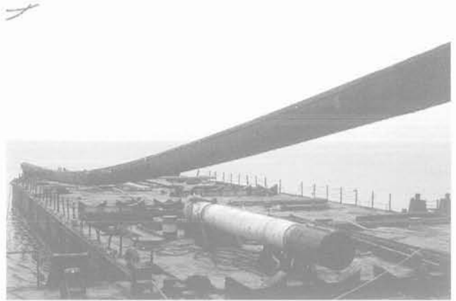
FIG. 7 Levage d'un pieu battu. Lifting of a casing for a driven pile.
