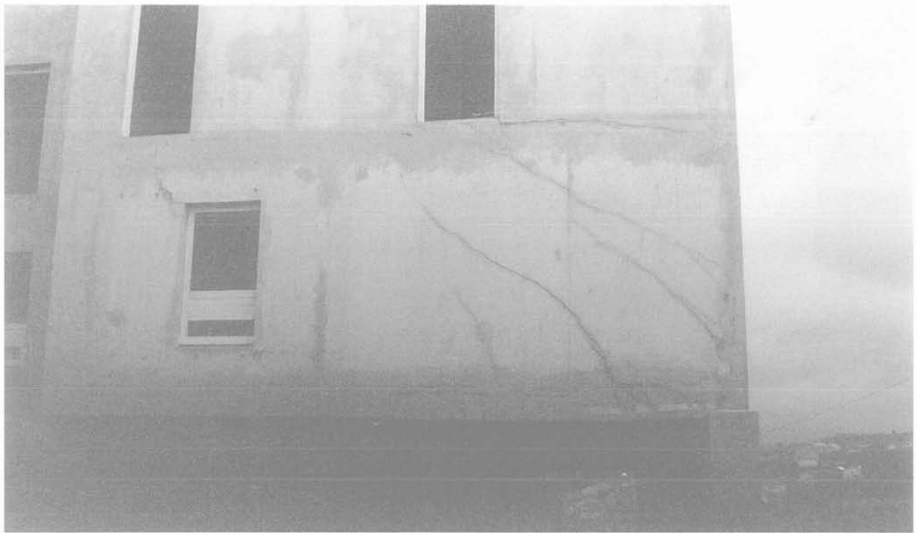
FIG. 2 Fissures caractéristiques de tassements différentiels. Typical cracks due to differential settlements.
