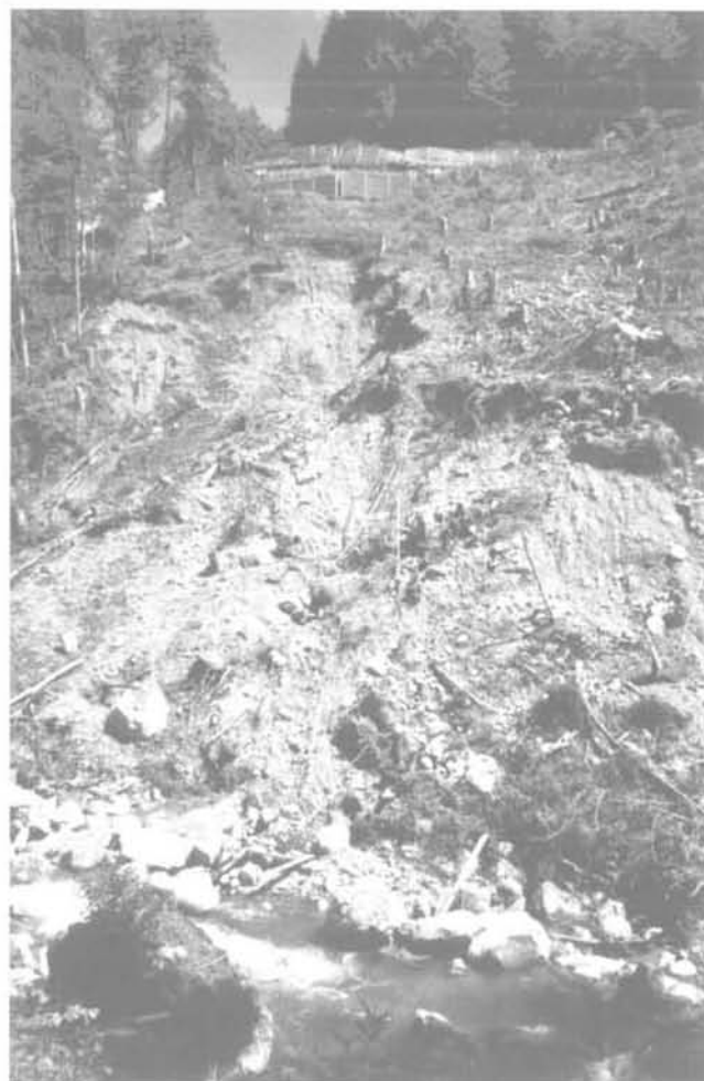
FIG. 5 Corps principal du glissement (photo : Bureau Maric). Main part of the landslide.
